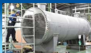
Factory (heat exchanger)
